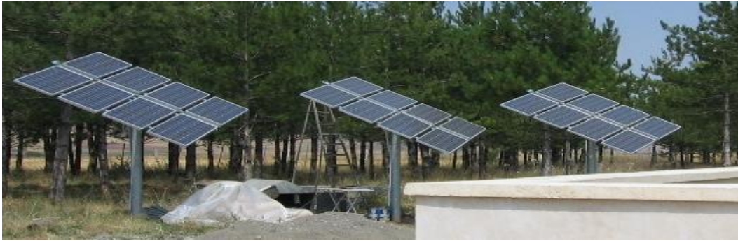
Figure 9 Image of Tilt PV module (Source: IJESI)
